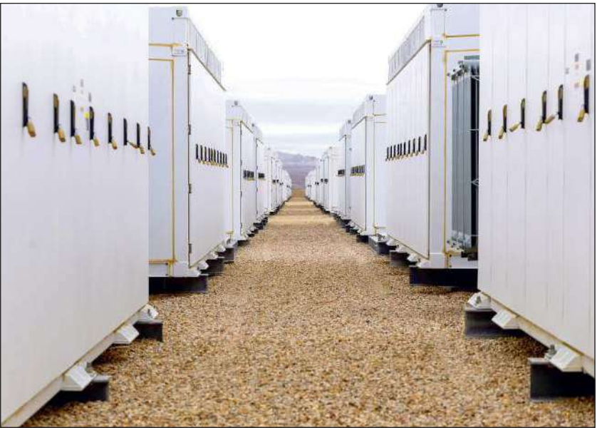
BATTERY SOLAR energy storage units at the LADWP’s largest solar and battery plant, the Eland Solar and Storage Center in Kern County.
